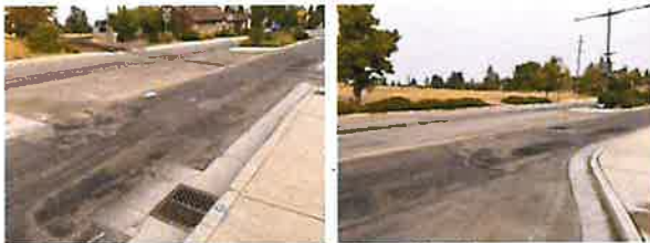
Examples of the condition of Spokane Street. The roadway is littered with rutting, cracking and settling.
