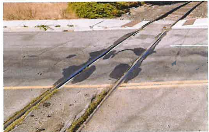
Design plans are complete that will replace this antiquated crossing with modern concrete planking.
