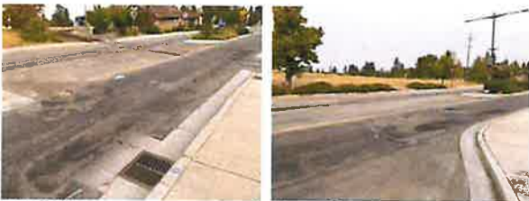
Examples of the condition of Spokane Street. The roadway is littered with rutting, cracking and settling.
