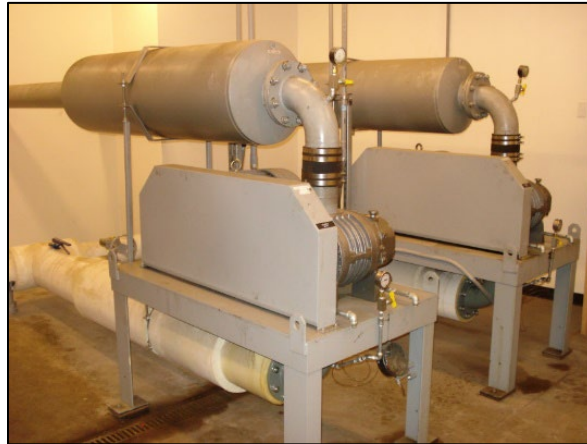
Figure 4-15 – UB2 Blowers (Tank 2)
