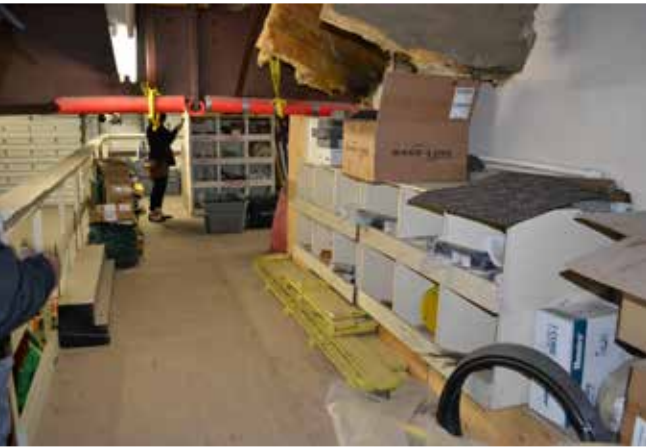
FIGURE 61. SHOP CEILING IN NEED OF REPAIR
