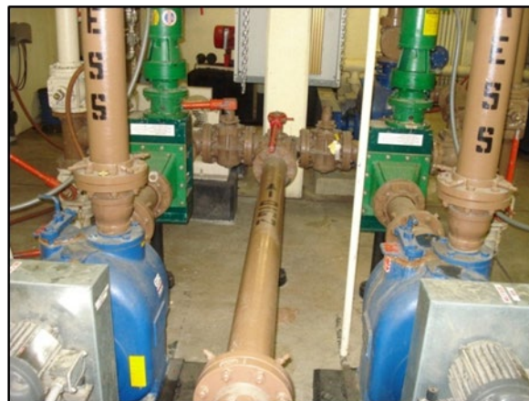
Figure 4-16 – Belt Filter Press Feed Pumps in UB-1 Serving Tank 1
