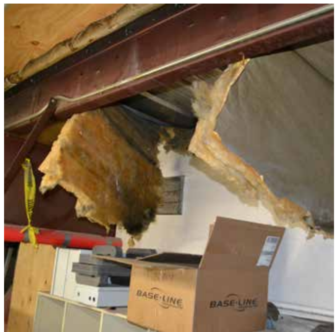
FIGURE 102. EXPOSED INSULATION AT THE PARKS M&O SHOP
