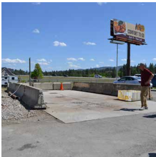
FIGURE 47. INADEQUATE STREETS WASH RACK
