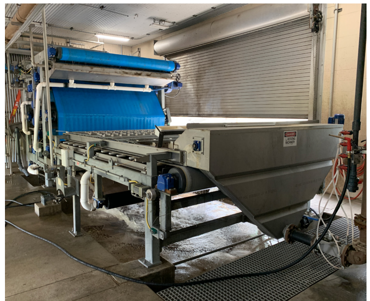
Post Falls WRF 2.5m BDP belt filter press installed approx. 2010.
