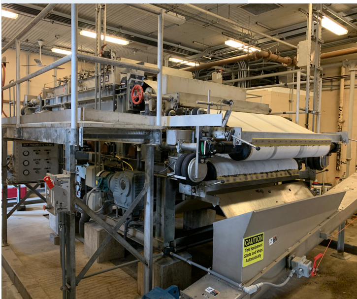
Post Falls WRF 1.5m Andritz belt filter press installed early 1990s.
