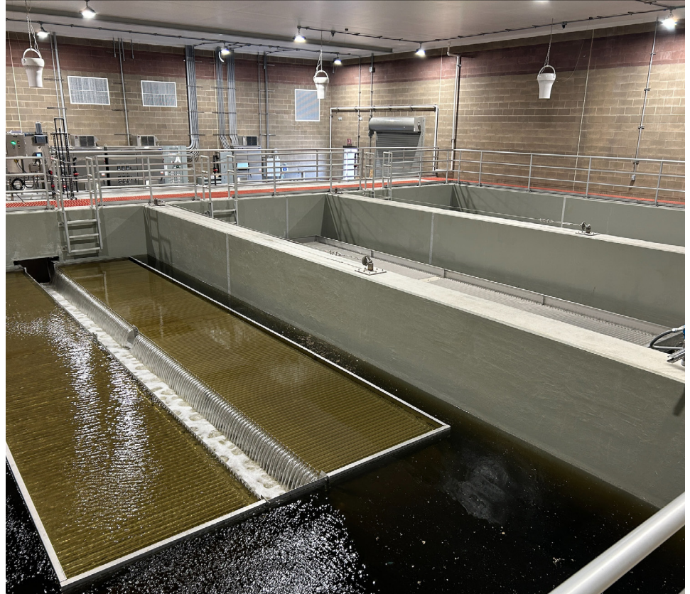
Post Falls tertiary plate settlers preliminary operations (no chemical addition), August 2024.
